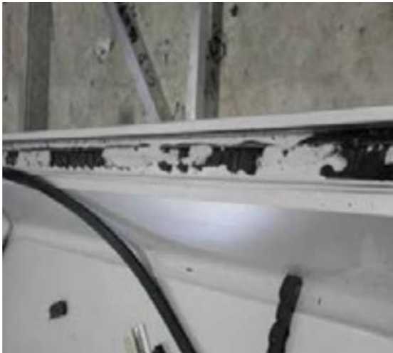
LARGE AREA OF SEALANT LOST ADHESION ON TO THE ALUMINIUM FRAME
