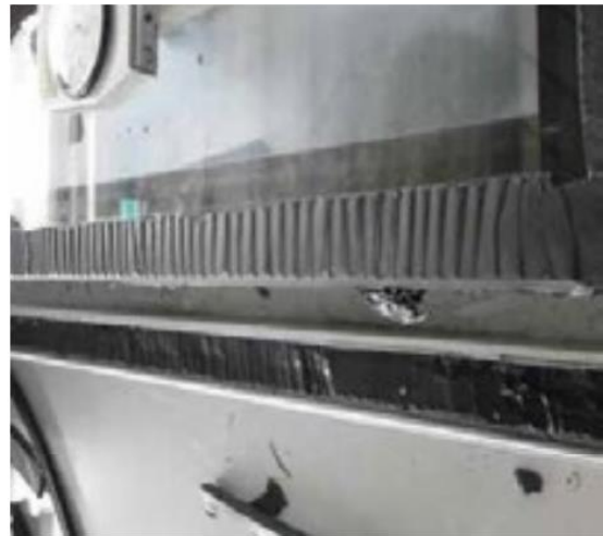
GOOD ADHESION WAS FOUND BETWEEN STRUCTURAL SEALANT ON TO ALUMINIUM
