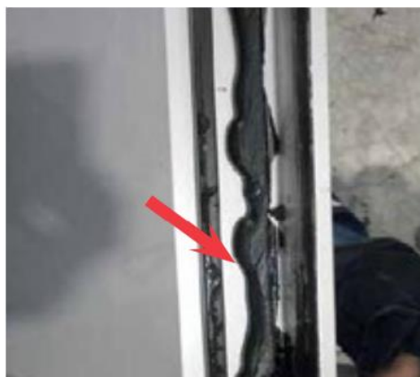
INCOMPLETE JOINT FILL
